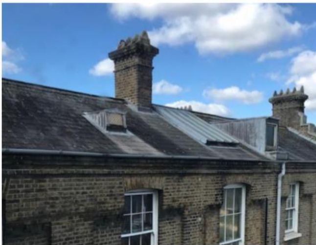
Figure 6: Photo of Decorative Vents and Rooflights.
